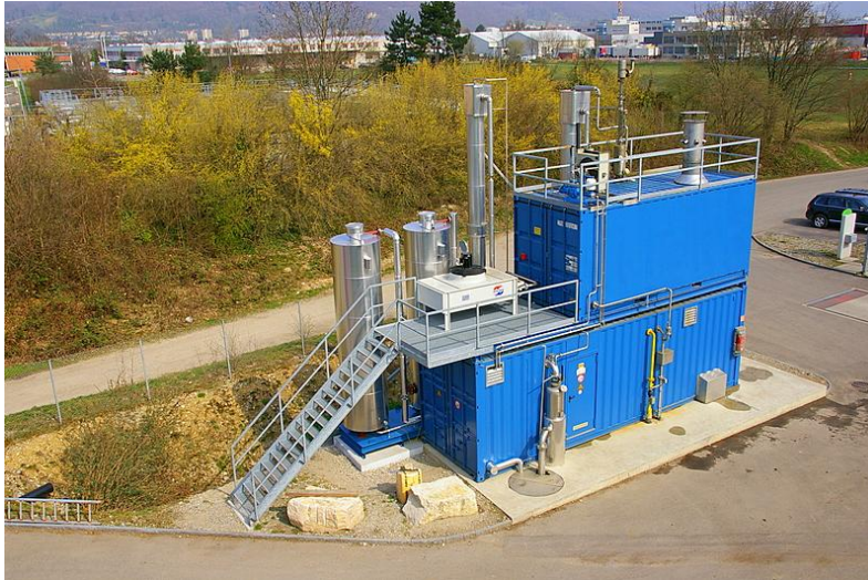
Fig. 3.2 Installation for biogas purification using glycol washing at the biogas plant in Pratteln (Source: Keller, Biopower Nordwestschweiz AG)
